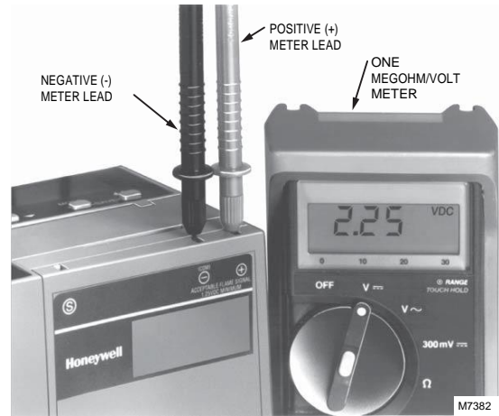
Fig. 11. Measuring voltage flame signal with 7800 Series controls.
