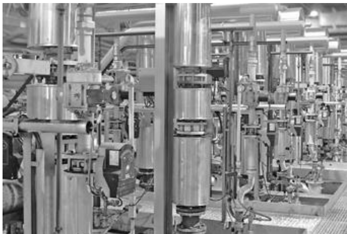
Walking beam furnace with overhead firing
