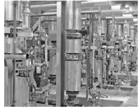
Walking beam furnace with overhead firing
