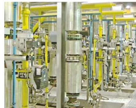
Walking beam furnace with overhead firing
