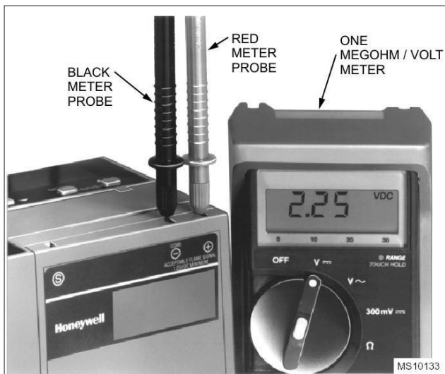
Fig. 11. Measuring voltage flame Signal with 7800 SERIES controls
