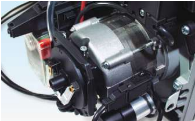
Pressure switch DL mounted on heating boiler
