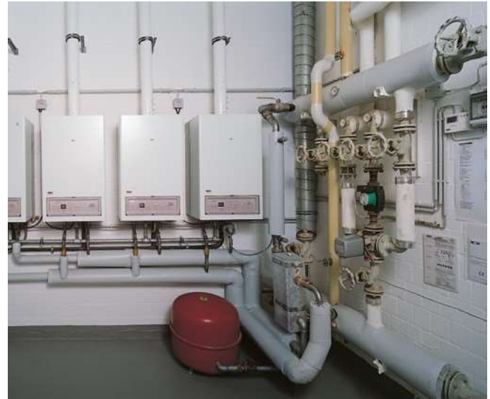
Heating boilers connected in cascade
